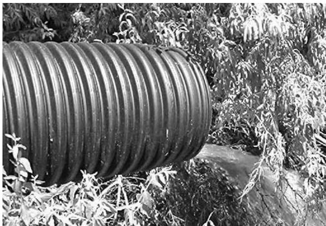
A field drain into the Bear River.
